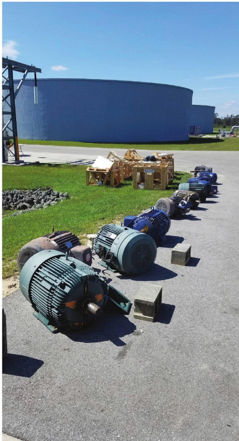
Damaged motors line the yard in the week after the storm.
