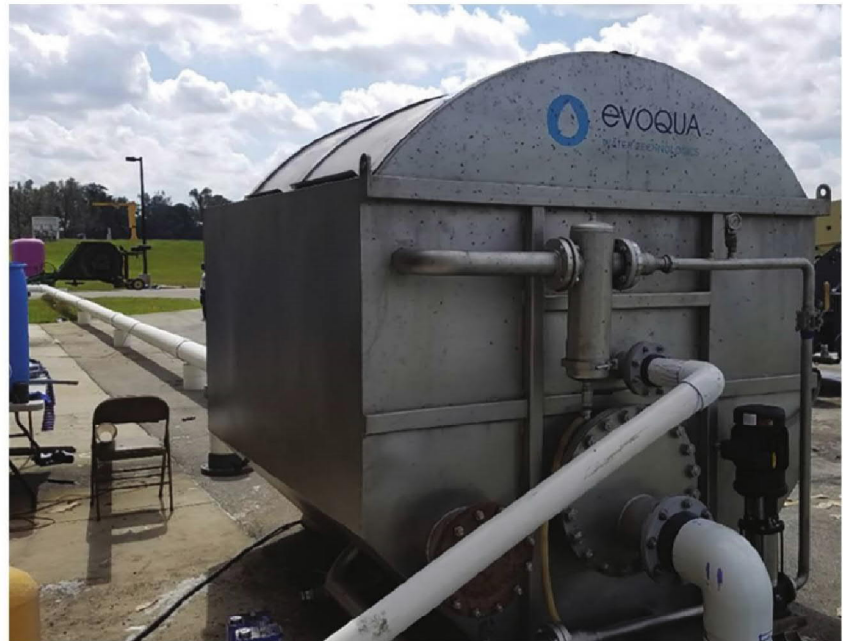
A portable disk filter unit arrived 10 days after the storm and enabled tertiary filtration to be restored on a long-term basis.
