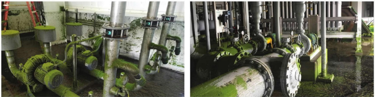
Floodwaters inside the plant reached more than seven feet above the 100-year flood elevation, causing extensive damage and leaving the plant completely inoperable.
