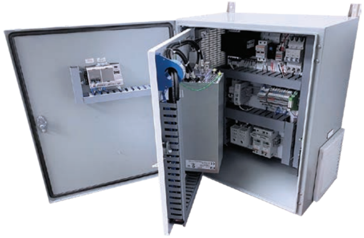
CAPAC system power supply controller (PSC)
