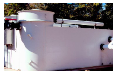
Deep-Bed Sand Filters
