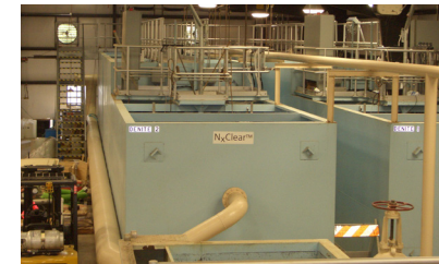
NxClear® Denitrification Filters
