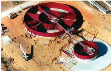
DAVCO™ Field Erected Treatment Plants
