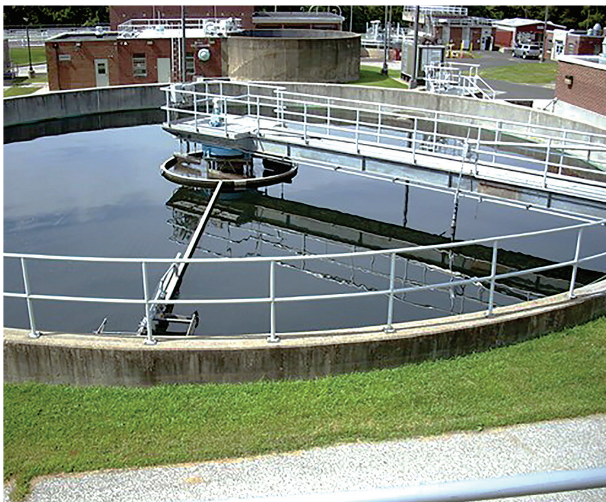
The Upper Gwynedd Township, Pa., WWTP has been using the process to handle wet weather flows since 2014.
