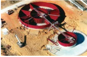
DAVCO™ Field Erected Treatment Plants
