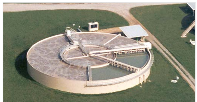
Dual Path Process 1 MGD installation in North Carolina
