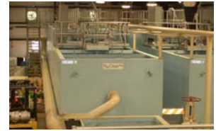
NxClear® Denitrification Filters
